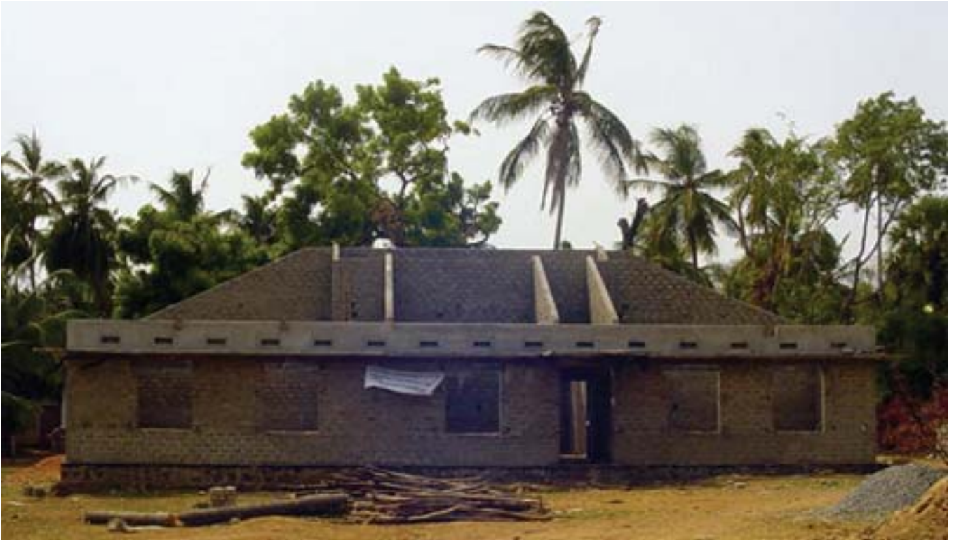
NJTACS sponsored Children's home is being built in Sambaltivu, Trincomalee. NJTACS will provide funds for long-term maintenane of this home.
